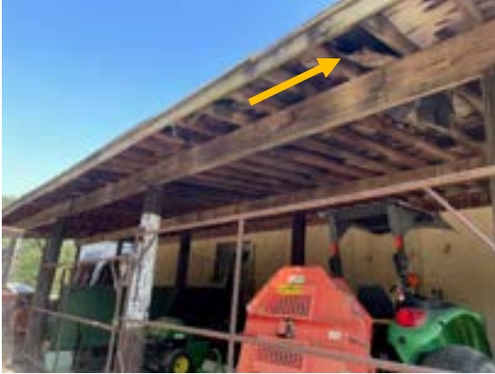
Photo 24 – Water Damage to Plywood
