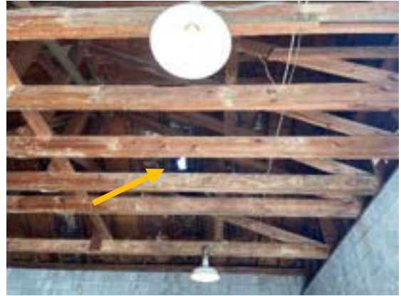
Photo 20 – Light visible thru Water Damage to Plywood
