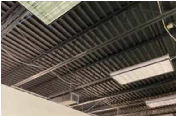
Photo 3 – Multipurpose Room Ceiling
