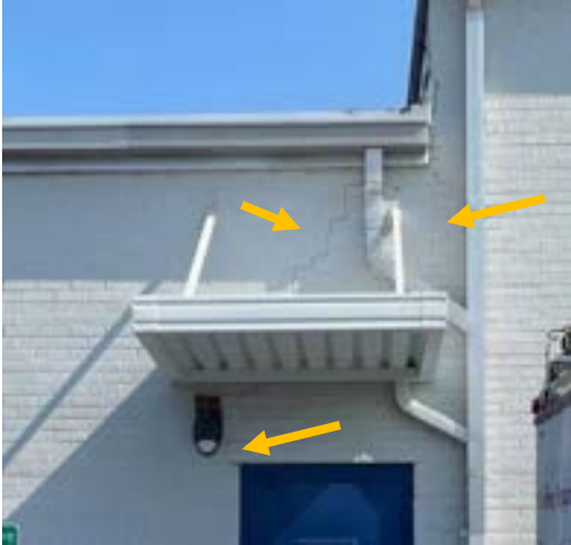
Photo 11 – Observed Exterior Crack
