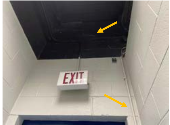
Photo 12 – Observed Interior Crack same location
