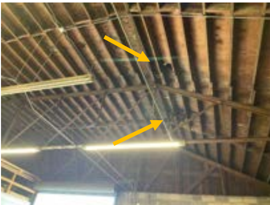
Photo 17 – Water Damage to Plywood
