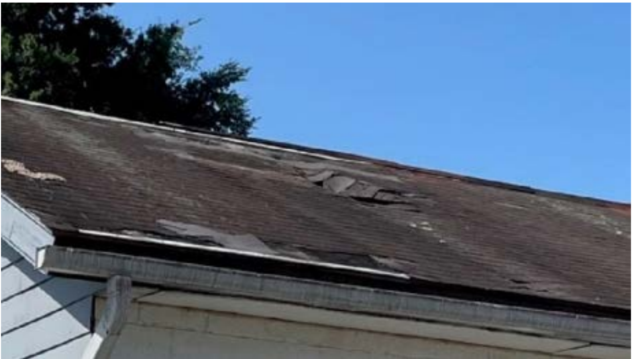
Photo 21 – Shingle Roof has Exceeded Life
