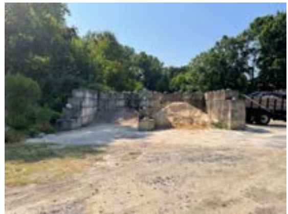
Photo 27 – Concrete Block Screen Storage Walls
